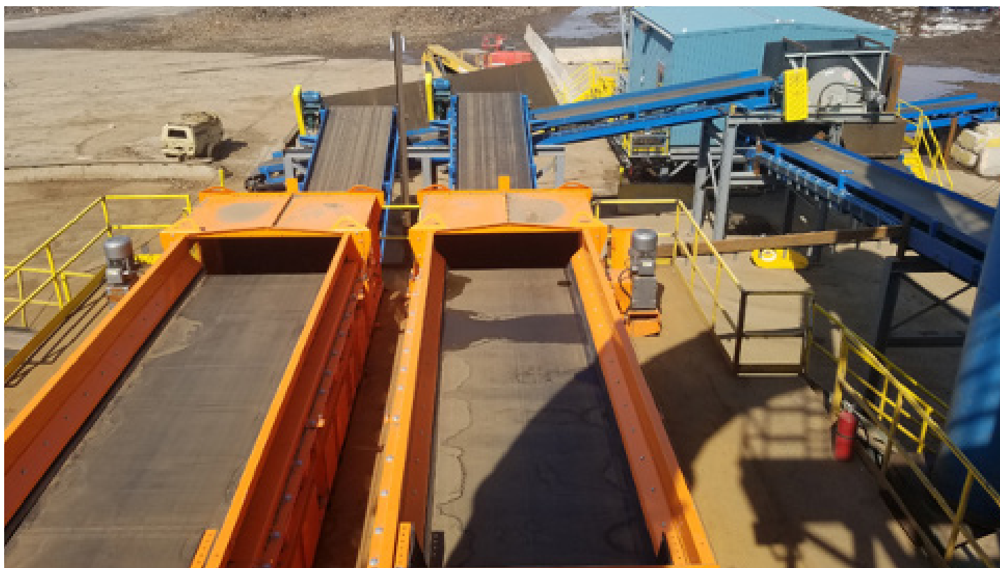
Shred1 Ballistic Separator installation with Polishing Drum
